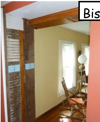
A look at the "cut through" identifies the structural beams that were erected in 1835 and 1870's. Examples of lathe work for plastered walls is provided to visitors to understand early construction of walls.
